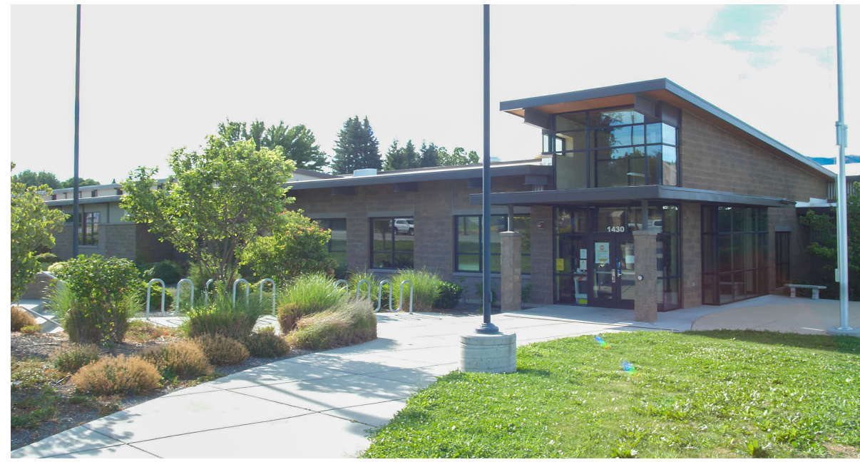
Grant Elementary School's expansion and renovation project – one of six projects funded in part by the capital levy approved by voters in 2016 and a $10 million grant – should be completed by August 12. School District.
