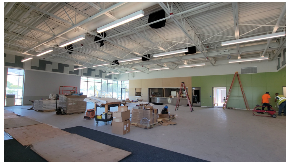
This new cafeteria and kitchen is part of the expansion and renovation project at Rock Island Elementary. The new annex also adds new classrooms and an adjacent parking lot.
